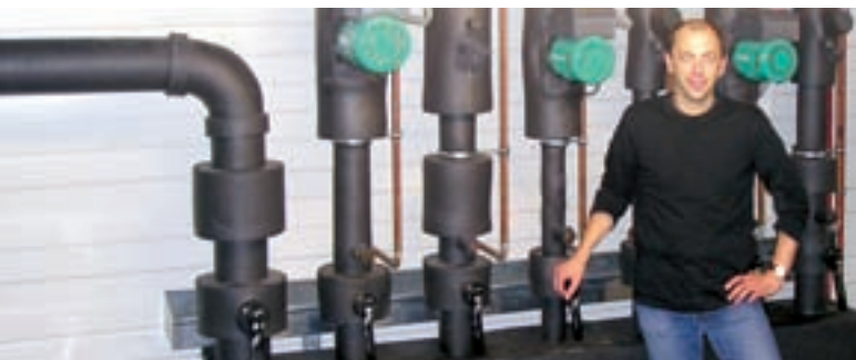
Jörg Holthöfer saves 120,000 kilowatt-hours of energy a year with the help of intelligent heating and cooling technology.
